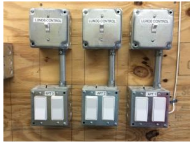
Controls outside of units
